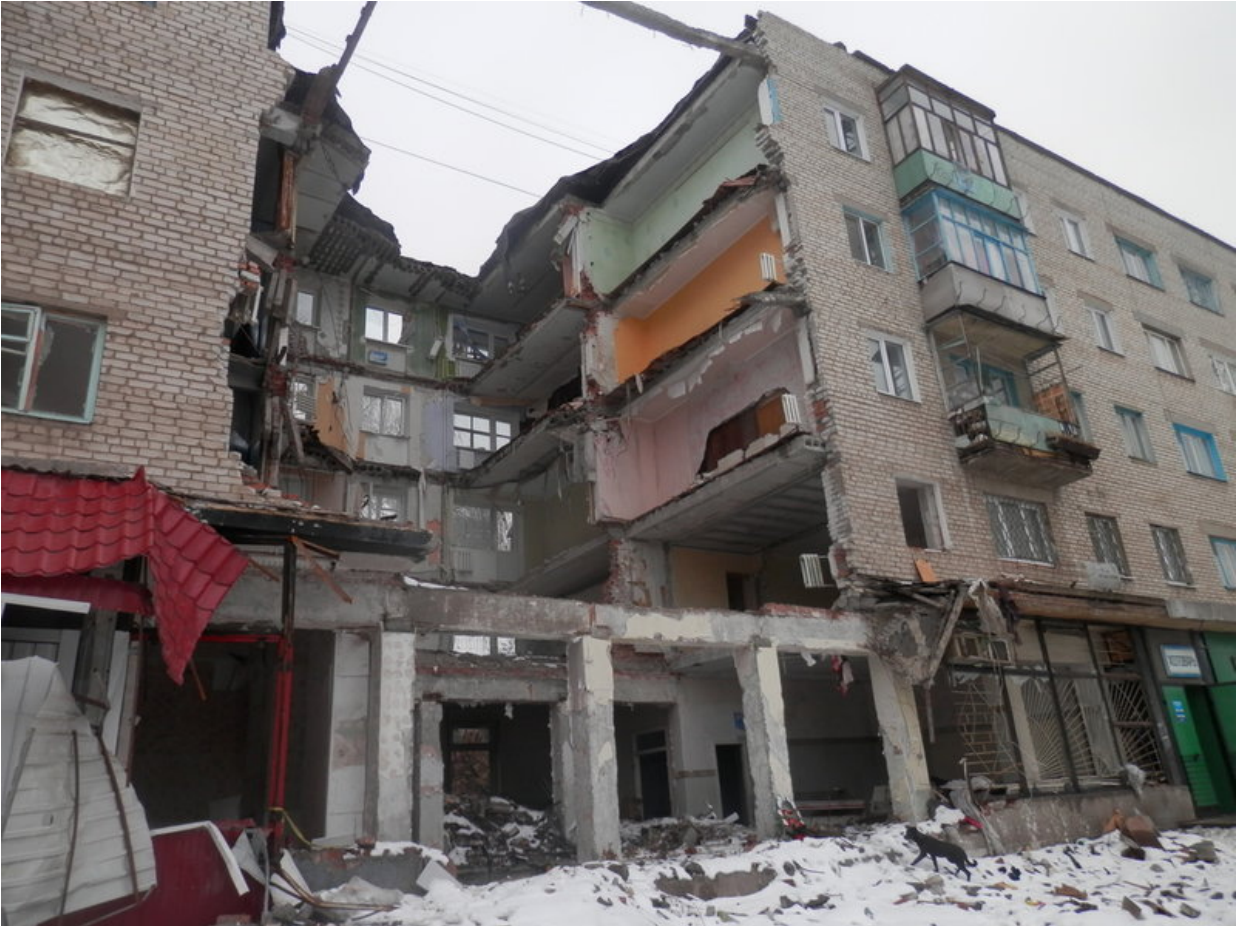
Apartments destroyed by shelling in Slovyansk (December 2014).
