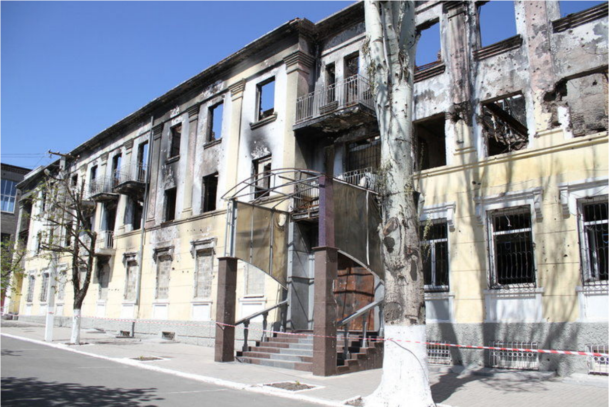
Ministry of Internal Affairs regional office damaged by fighting when the Azov battalion re-captured Mariupol in the first phase of the war (April 2015).
