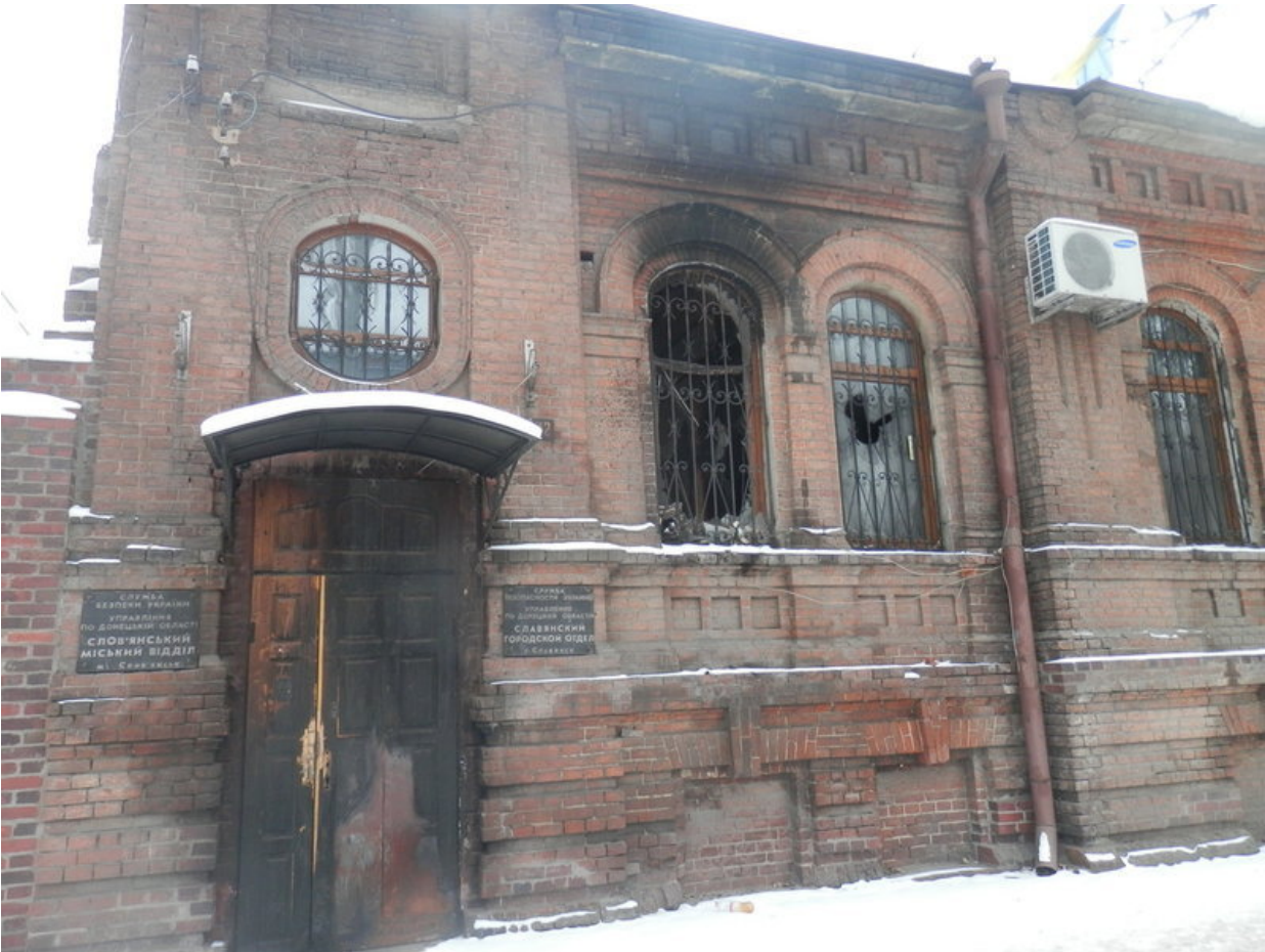
SBU regional office in Slovyansk damaged by fighting when Igor Girkin's Russian forces captured the city (December, 2014).
