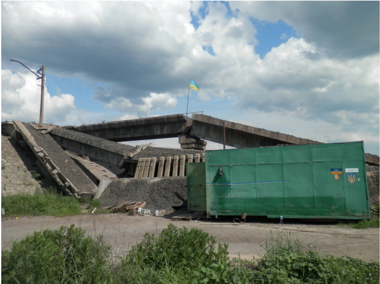
Motorway bridge on the highway to Donetsk blown up by Russian and separatist forces as they fled advancing Ukrainian forces (Pisky, March 2016).
