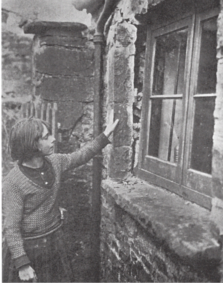
Gap by a window of a school in Wales
