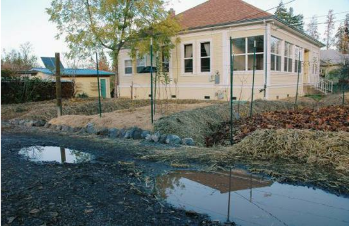
Newly installed earthworks including swales, berms, permeable pathways, French drains, and keyhole planting in this Willits, California yard. The standing water seen in the foreground was common throughout the site before the earthworks, compost, and mulch were installed. Posts for trellising the mini-food forest can be seen where the lawn once was. In the background is the downspout leading to the water storage under the house and to the left the garage/guest room features trellises for vertical gardens in front of it. Design by Maximillian Meyers of the Mendocino Ecological Learning Center. PHOTO BY MAXIMILLIAN MEYERS.
